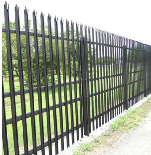
Steel Security Fence
